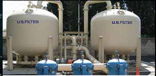
Tanks for an ion exchange perchlorate-removal process treat groundwater at a NASA-funded water plant.
